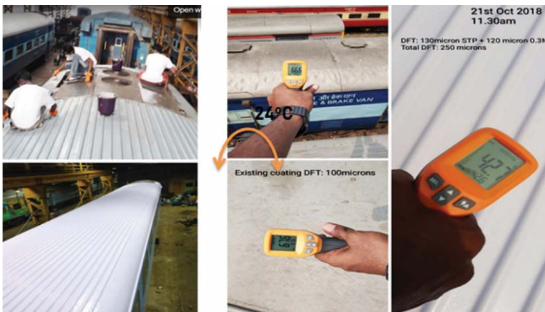
Fig. 3: The application of SHRC coating on the roof of an air-conditioned railway compartment reduced the temperature by 24 °C which can substantially reduce the electricity consumption of the AC.
