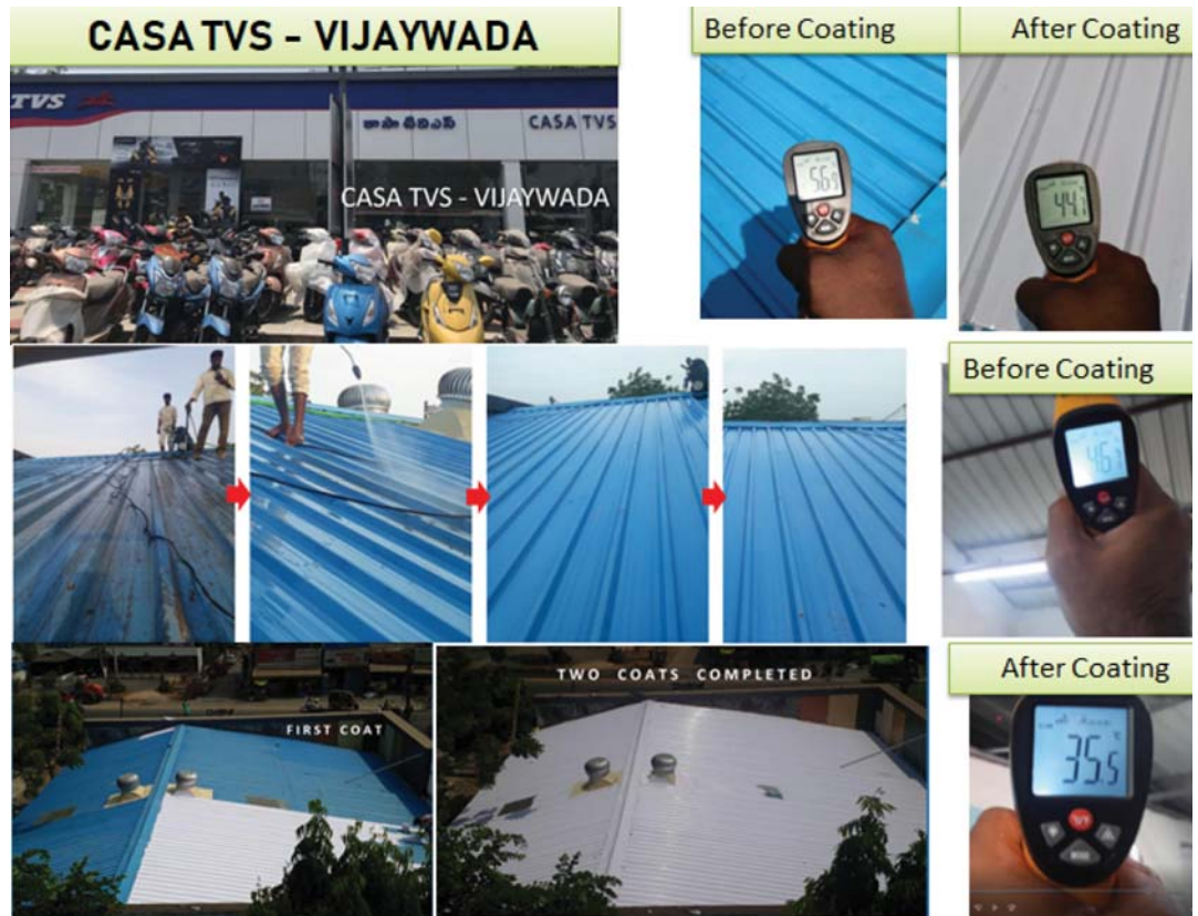
Fig. 1: An example showing the cooling effect of 12^\circ\text{C} on a steel shed roof in Vijaywada.
